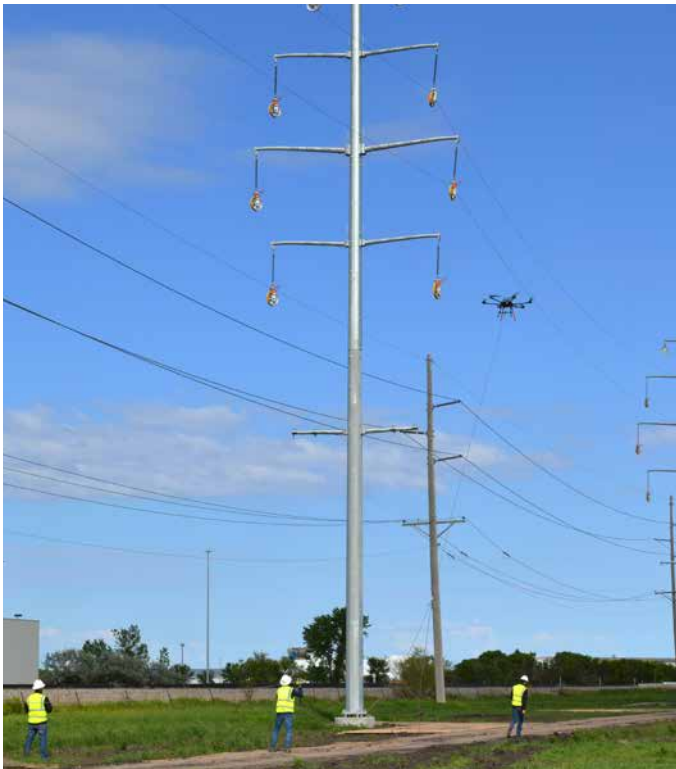
✦ Xcel Energy recently completed a five-mile, 115-kilovolt transmission line within the City of Fargo. The line provides increased reliability of electric service in the Fargo area by reducing overloads on neighboring lines and transformers. A drone was utilized for the first time on this project to assist in stringing the lead line for the conductor. Photo courtesy of Xcel Energy.
